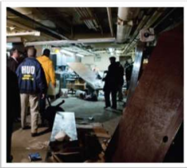
Secretary Donovan views storm damage in a basement at the Booker T. Washington Public Housing Complex in Jersey City, NJ (Official White House Photo by Sonya N. Hebert)
